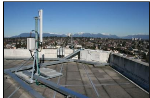
Antenna Attached to Roof of Existing Building
