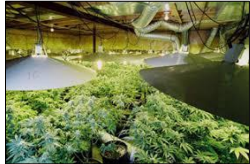
Grow lighting is exempt from Washington State Energy Code Requirements.
